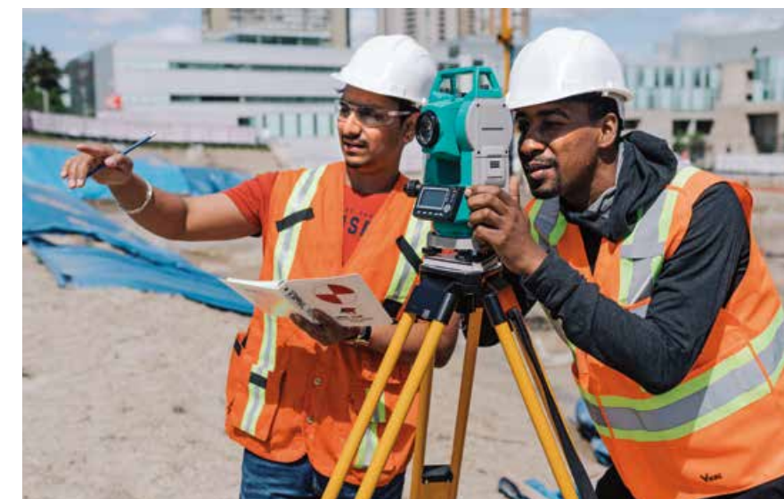
PICTURED ABOVE: Civil Engineering Technology students learn to survey the new Centre for Innovation, Technology and Entrepreneurship (CITE) construction site at Newnham Campus.
